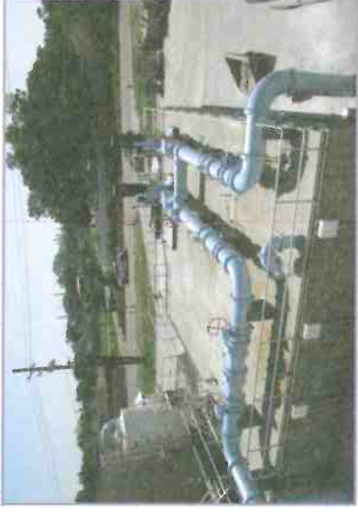
Clear Well Pump Station
