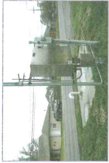
SCADA Remote Station
