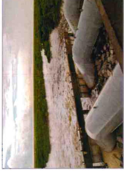
Pump station discharge into central wetlands
